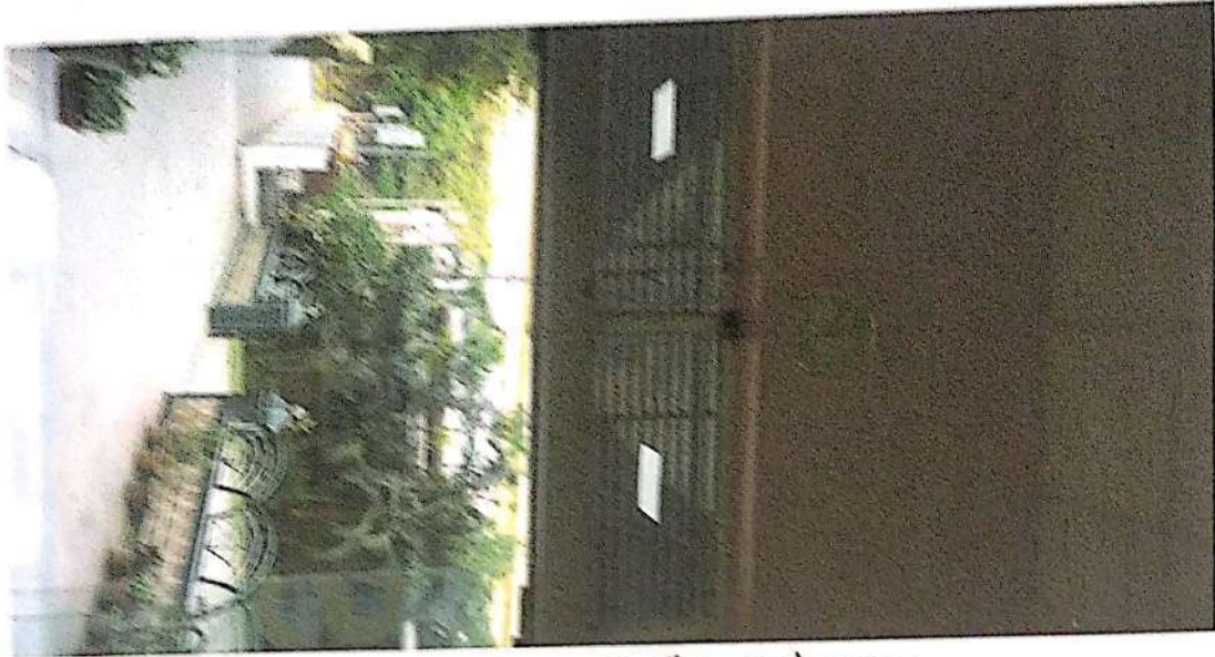
CCTV camera main Entrance
