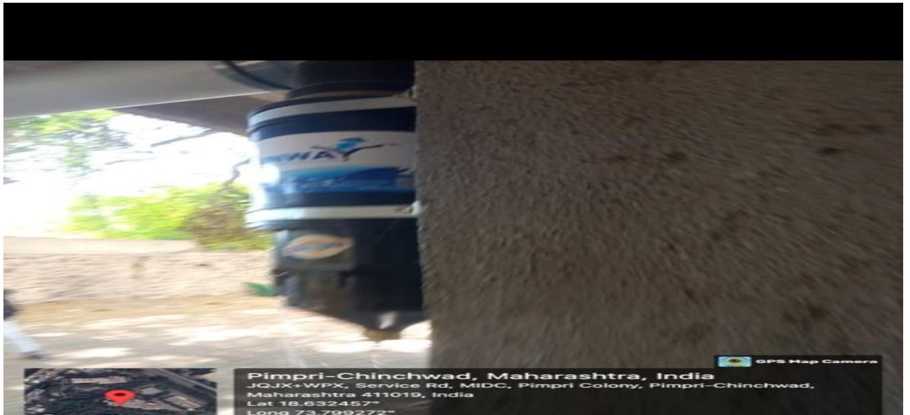
Rainwater Carrying Pipe and Filter
