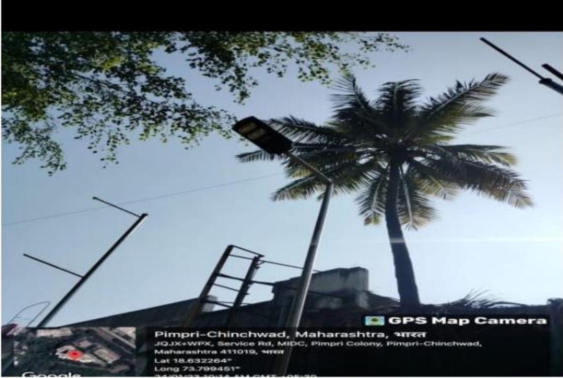
Power Saver Equipment's installed in the campus.
